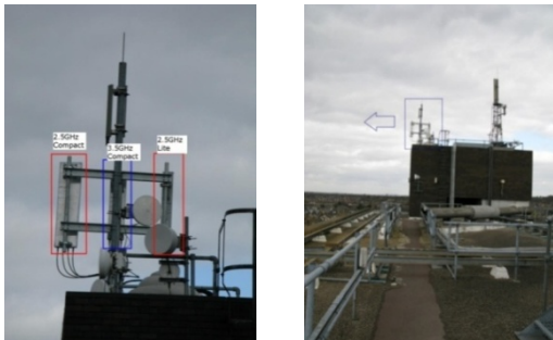
Fig. 2 Close-in view from the back of the WiMAX antennas as arranged on the supporting frame (left) and view from the opposite end of the roof (right)
